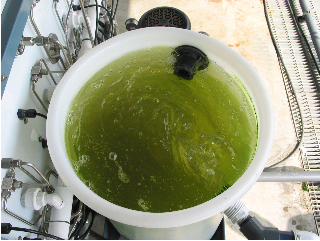
Figure 9. WB test unit feed water tank. 1032 hours of operation. Green color is the result of algae contamination.
